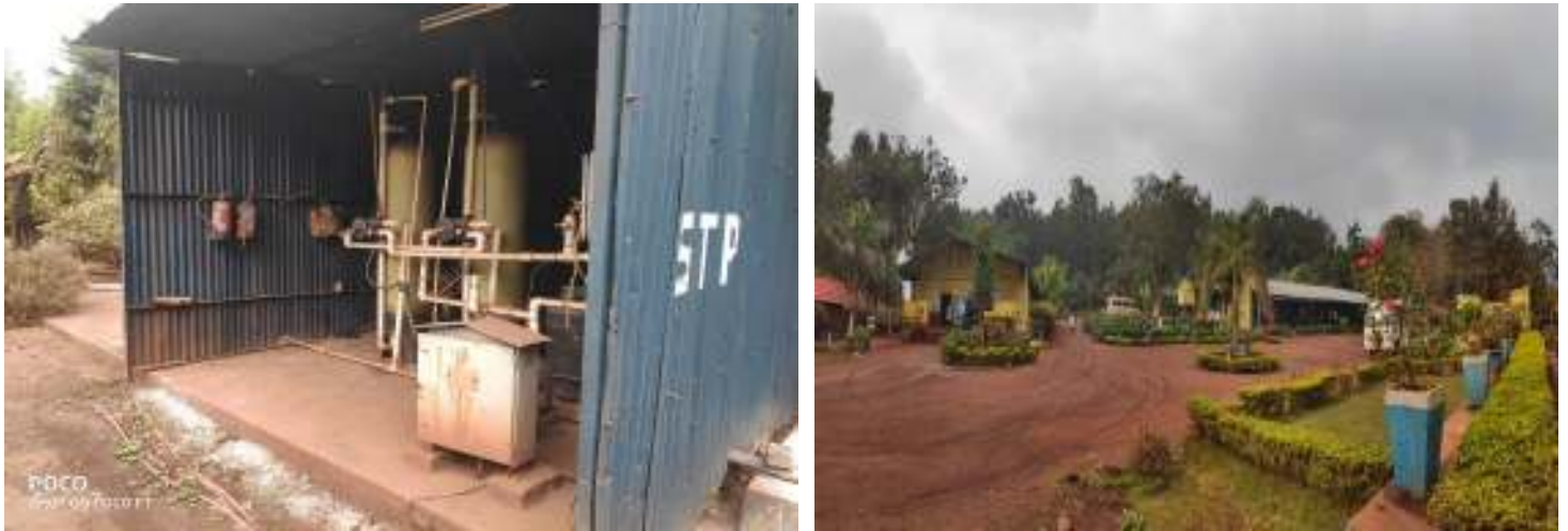
Photo-11: STP for treatment of Domestic Waste Water (Ultra Filtration Unit) & its utilization in green belt development
