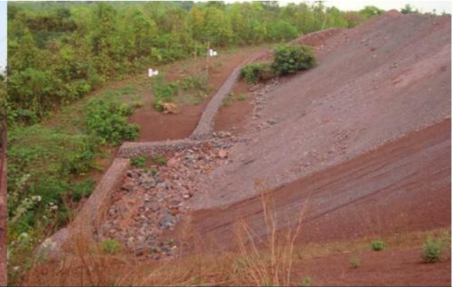
PHOTO # 1-C: SHOWING RETAINING WALL ALONG WITH GARLAND DRAIN ALL ALONG THE DUMPS
