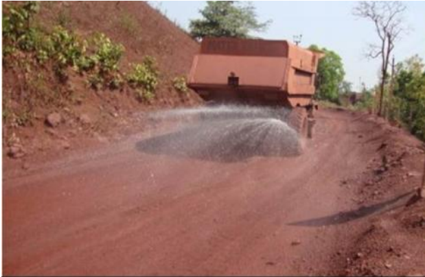
PHOTO # 1A SHOWING THE WATER TANKER ON HAULAGE ROAD FOR DUST SUPPRESSION
