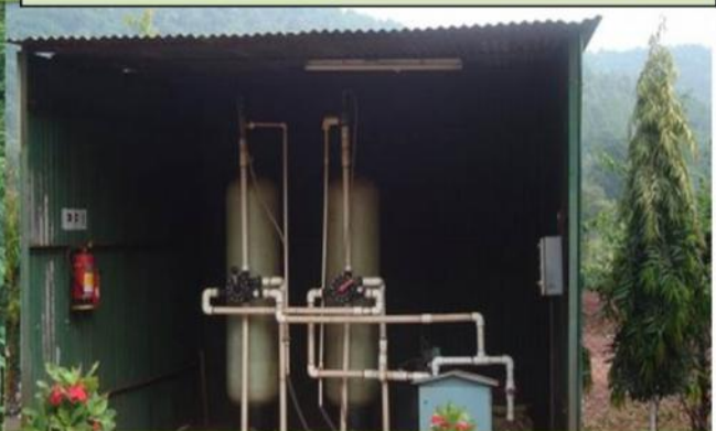
PHOTO # 8 : SHOWING THE STP FOR TREATMENT OF DOMESTIC EFFLUENTS
