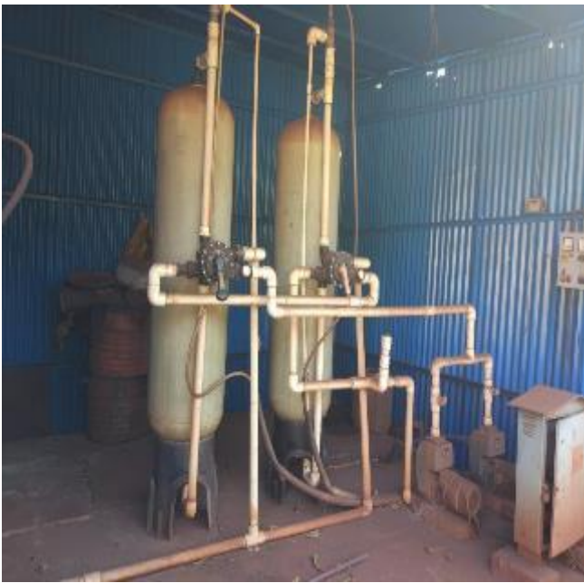
Pic 9- Sewage Treatment Plant
