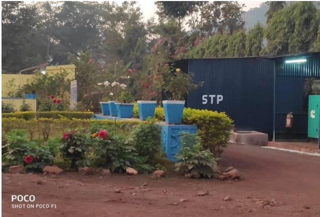
STP for treatment of Domestic Waste Water
